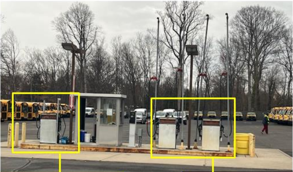
(1) Gasoline Dispenser Removed and Replaced with new as well as all accompanying ancillary equipment.
